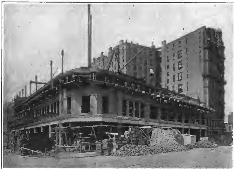
BUILDING THAT IS SAID TO BE THE LARGEST AUTO SALESROOM IN THE WORLD.
